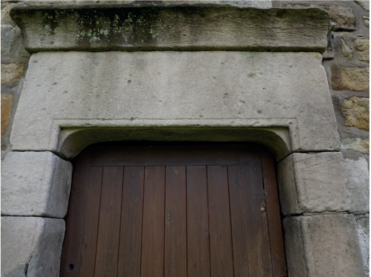
Figure 9 Mitchell House, Thorpe, lintel.
